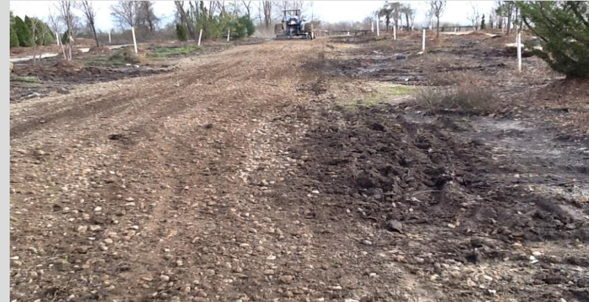
Before: Untreated dirt road with severe rutting
